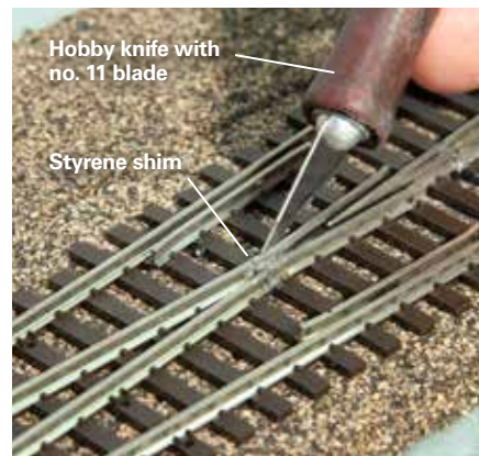
Fig. 3 An easy fix. To prevent the rails from closing up due to expansion or movement, Larry installed styrene shims in the gaps. He trimmed them to match the profile of the rails with a no. 11 blade.
