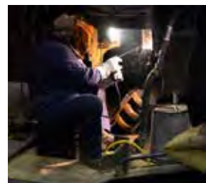
Working at the Barrie-Collingwood shop in Utopia, Ont., an LDS mechanic finishes up a new drawbar installation on GP9 1001.
