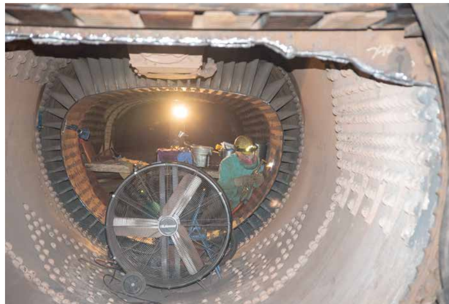
Looking down the barrel of the long boiler from the smokebox end, and with both front and rear tube sheets removed, boilermaker Jimmy Thompson uses a cutting torch to remove a staybolt.
