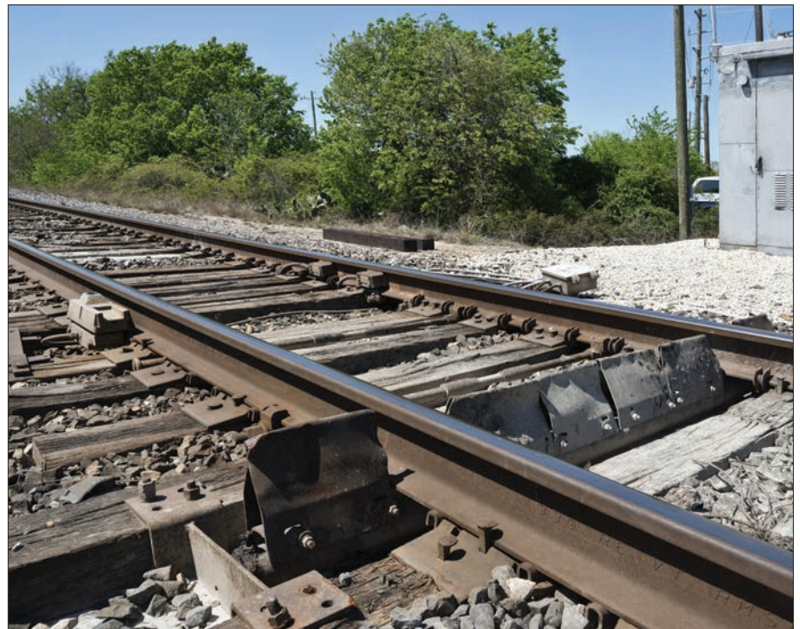
This BNSF installation in 2014 includes a dragging-equipment detector (paddles in foreground) as well as a hot-bearing detector (outside the rail at left) and a pair of wheel counters (inside the rail opposite the bearing detector). Tom Kline
