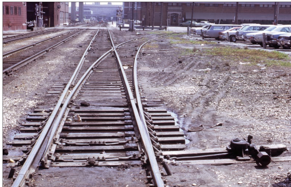
The split-point turnout has two moving rails (points), with ends tapered to match the outside (stock) rails. They allowed higher speeds and eliminated the alignment issues of stub switches. Gordon Odegard
