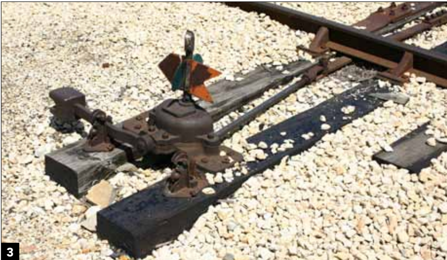
3 Ground throws are found along yard and industrial tracks.
