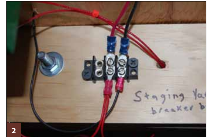
2 Label all wires, terminal strips, and connections. You can make notes directly on the benchwork.
